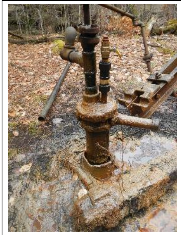
Orphan Well Oil Spill, Warren County, Pennsylvania The "Confluence Well"
